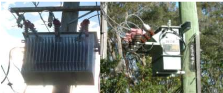
Fig. 10 TRANSFORMER TURN RATIO TEST
